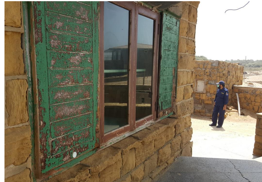
The timber work on the seaside was worst
