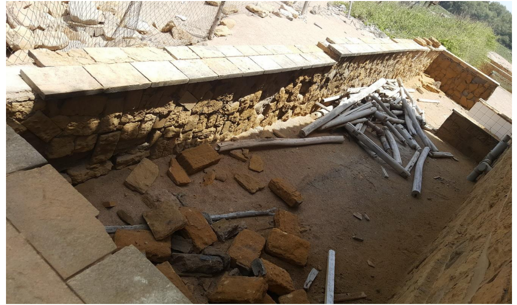
The BBQ area was never completed
