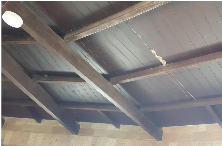
Lighting was poor, timber ceiling was painted brown
